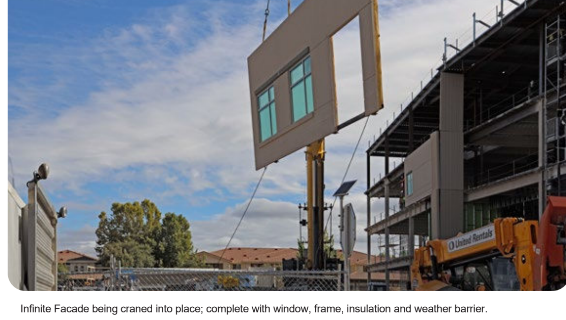
Infinite Facade being craned into place; complete with window, frame, insulation and weather barrier.
