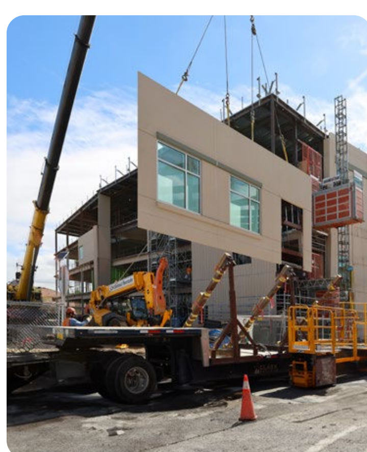
Infinite Facade being lifted off the truck and ready to be erected on the building.
